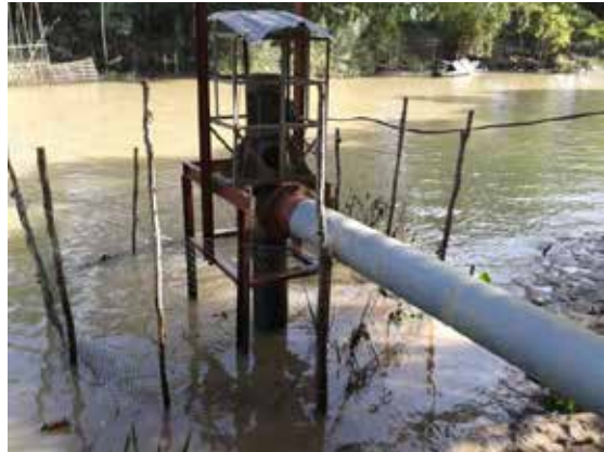
Figure 3: Small electric pump in VMD
